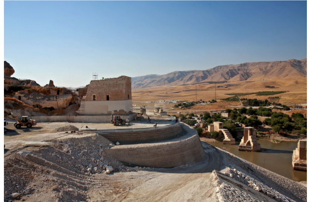
Construction work on the wall to protect the ruins of the citadel of Hasankeyf, which stands above the cliff, from the arrival of the waters of the lake. (2019)
