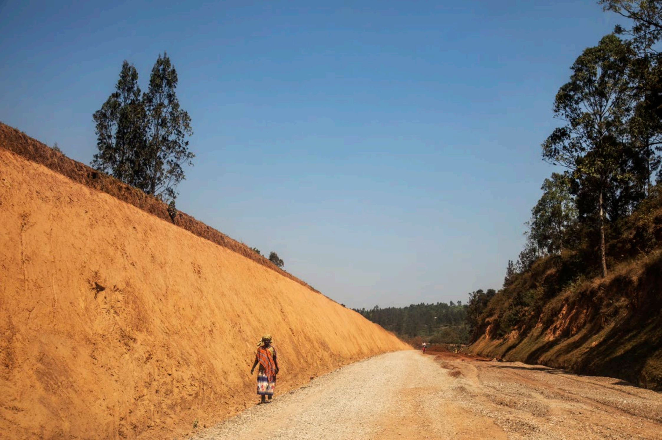
One of the new roads built by Chinese companies in the Gatsibo district.
