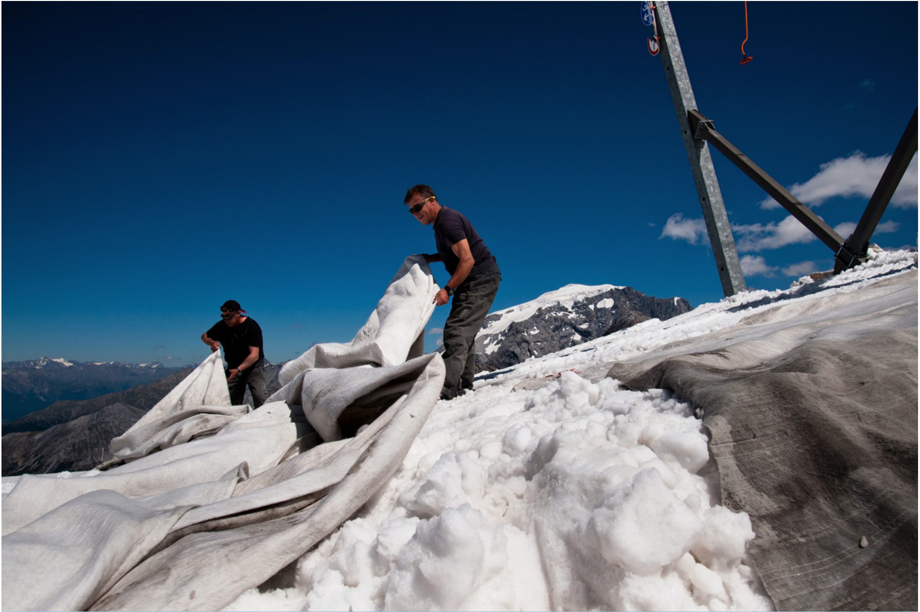
The Stelvio Pass (Italy), workers arranging special tarpaulins near some ski lift masts. These tarpaulins are crafted by the Italian company Edilfloor, and can help reduce the melting of snow and ice. In 2022 summer ski lifts on the Stelvio glacier did not open, for the first time.
