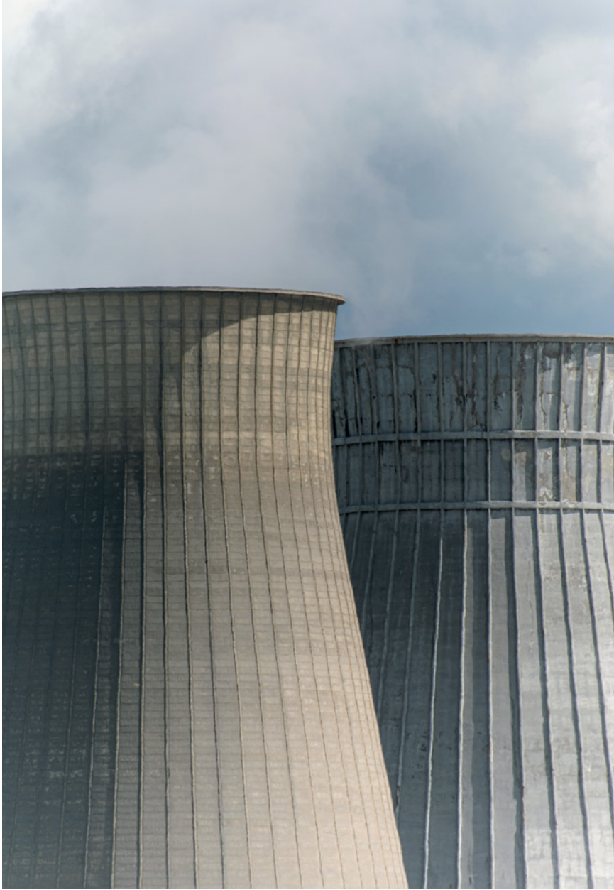
Rosignano Solvay (Italy). The cooling towers at the main plant.
