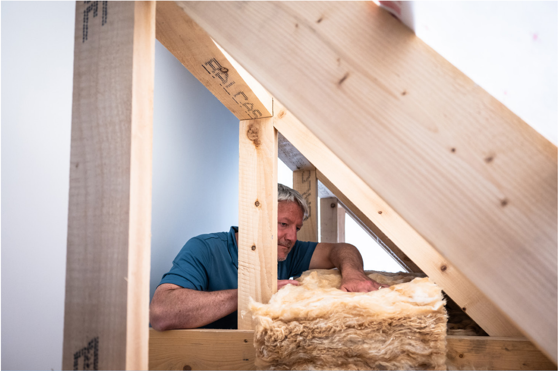
Templemore (County Tipperary, Ireland), Derry O'Donnell, ECTC Development Coordinator, checks the insulation quality at Sola Energy Solutions. Sola works alongside ECTC on the energy efficiency of many homes in County Tipperary.
