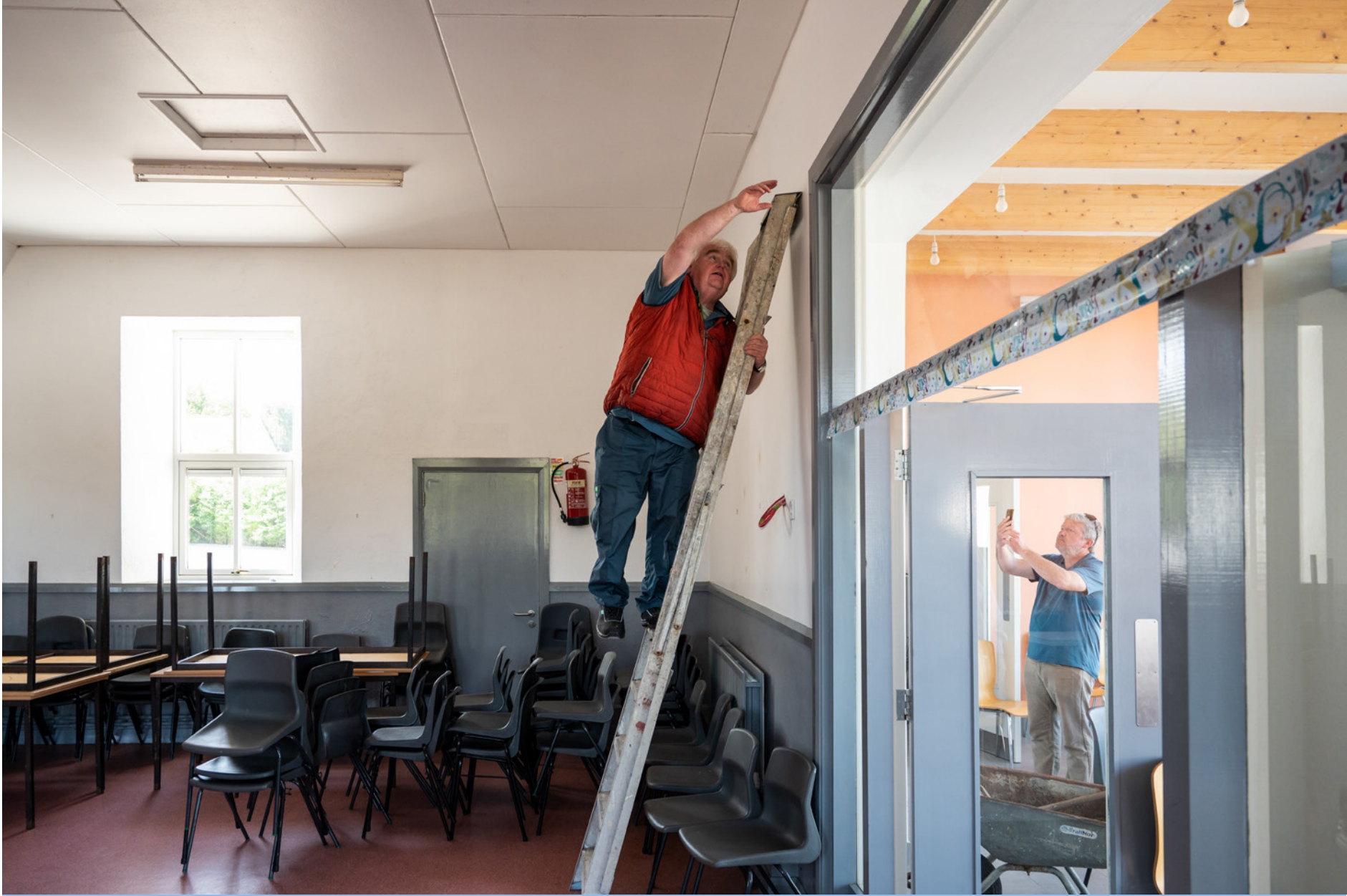
Rear Cross (County Tipperary, Ireland), Noel McMahon working inside the Community Hall. Noel is a member of the Kilcommon Rearcross Energy Team and the ECTC, which renovated the building and made it more energy sustainable.
