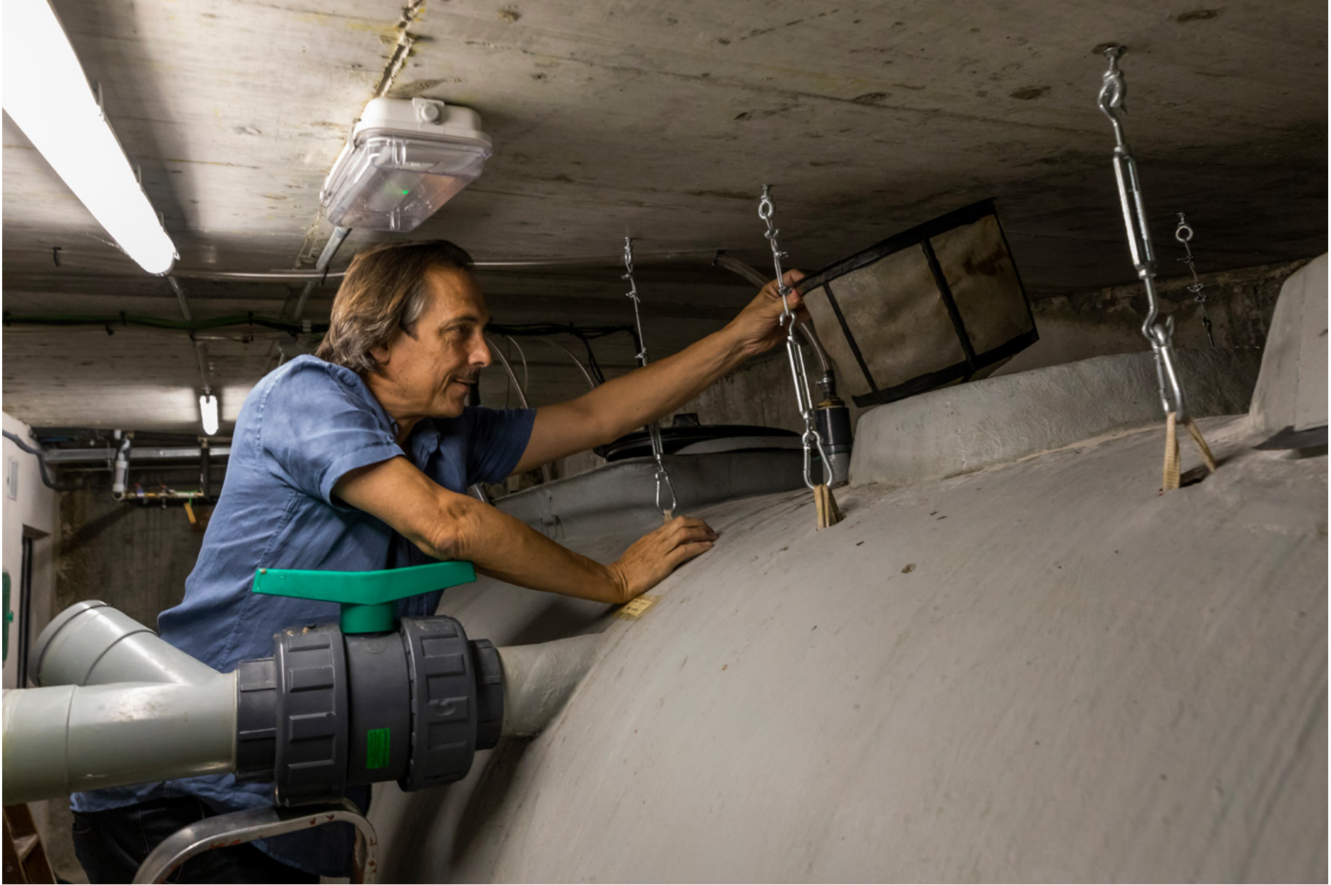
Madrid (Spain). Iñaki Alonso, one of the architects who designed the Las Carolinas building, where he lives with 16 other families from the Entrepacios housing cooperative. Here he is seen removing the filter from the cistern where sewage and rainwater are collected prior to being purified and reused for toilet drains and watering plants.
