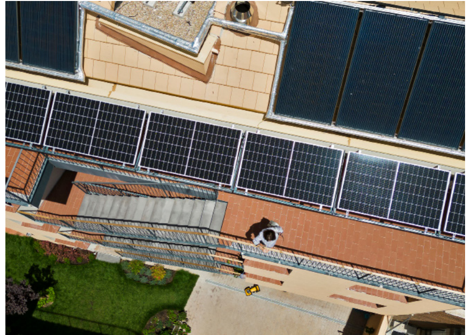
Madrid (Spain). Photovoltaic panels on the roof of the Entrepacios co-op building in the working-class Las Vallecas neighborhood on the southern outskirts of Madrid.
