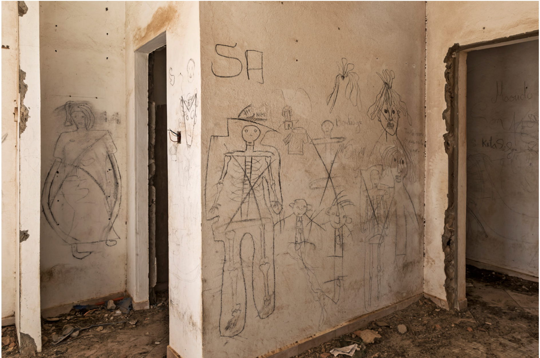
Senegal, St. Louis region - The walls of a house in the village of Pilote, on the edge of the Parc National de la Langue de Barbarie, destroyed by the sea, have become a blackboard for children's drawings. This village and several others that once stood along the mouth of the Senegal River, after the opening of the canal built to drain the waters from St. Louis, found themselves exposed to the fury of the sea and several houses were destroyed.
